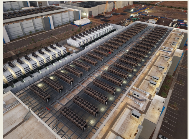
Roof of a data center featuring cooling towers and backup generators, November 2025 by Rsparks3
