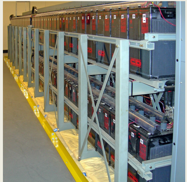
A bank of batteries in a large datacenter, used to provide emergency power until diesel generators can be started. 2007. Source: Jelson25
